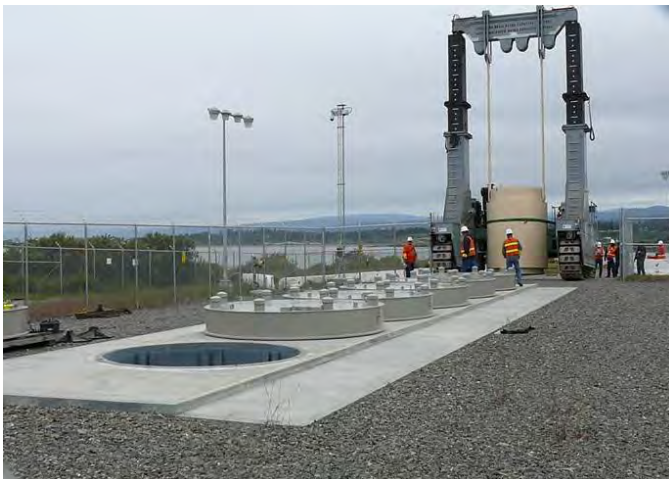
Underground Storage Modules at Humboldt Bay
