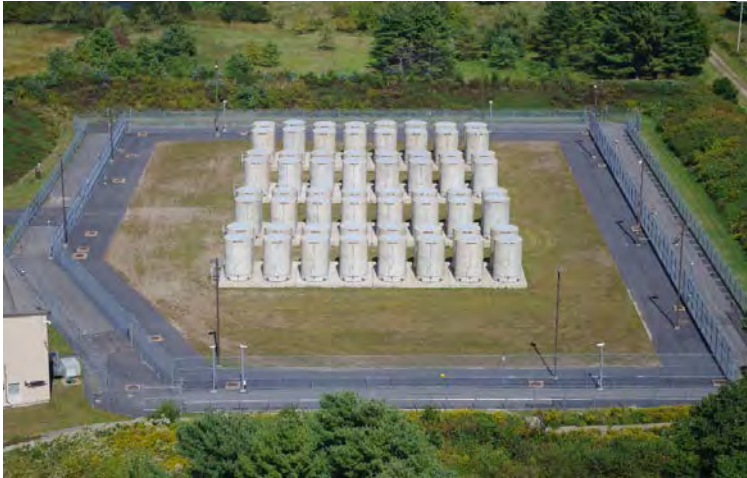
Vertical Concrete Casks (VCCs) Deployed at 9 Sites
