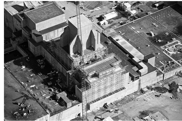
Workers prepare for roof installations on portions of the P Reactor at Savannah River Site that are expected to remain after facility decontamination and demolition efforts.
