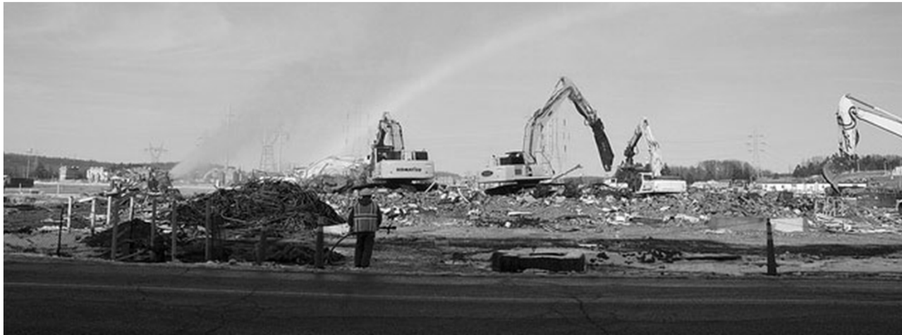
Recovery Act workers demolished a cooling tower complex and nearby electrical switchyard that together spanned more than 40 acres on the northeastern portion of the Portsmouth Gaseous Diffusion Plant.
