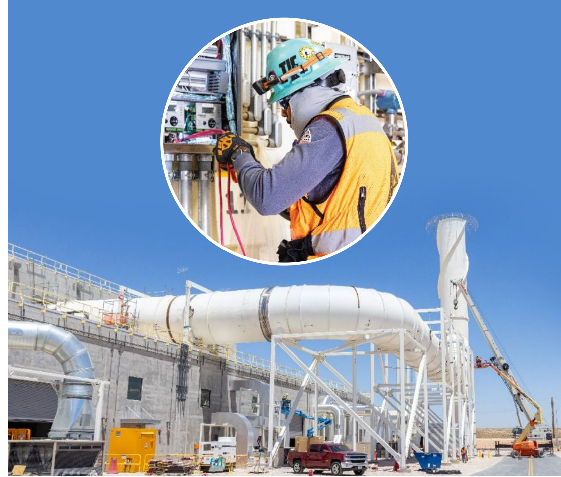
Above: Equipment testing during SSCVS commissioning Below: SSCVS final large duct work installation
