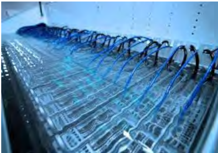
Liquid Immersion Cooling (Image Source:)
